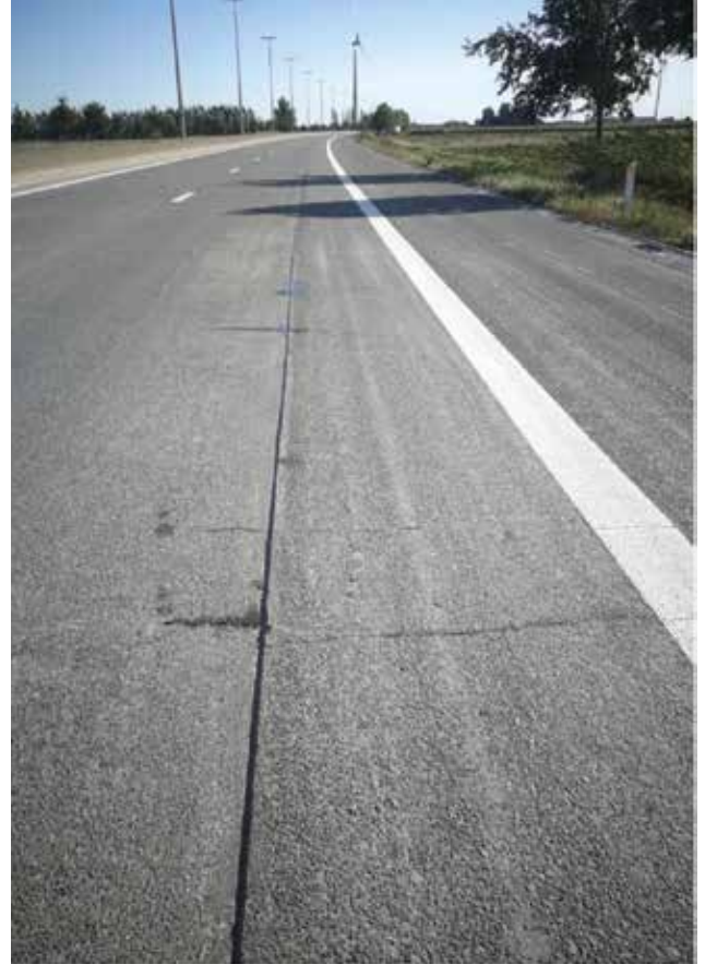
Figure 1: Regular crack pattern with the application of the saw cut as crack initiation (E34 – Kaprijke)
